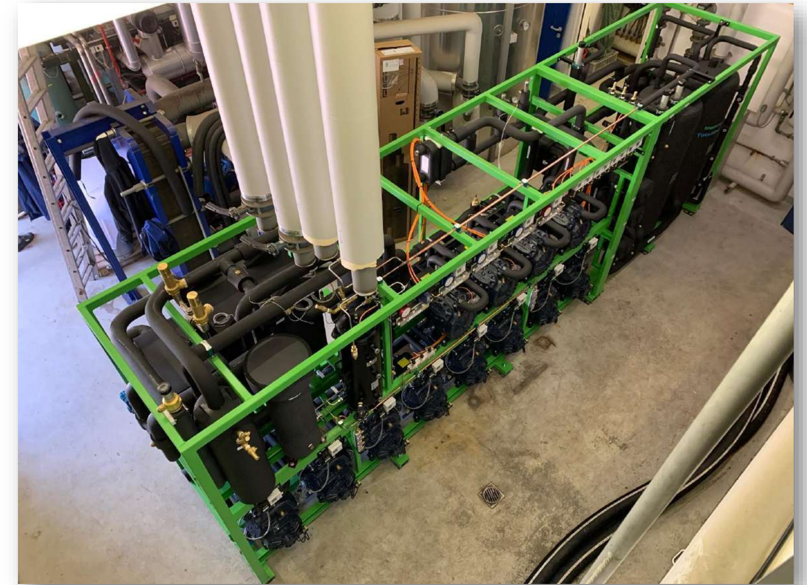
Compressor rack positioned instead of old reversible heat pump
